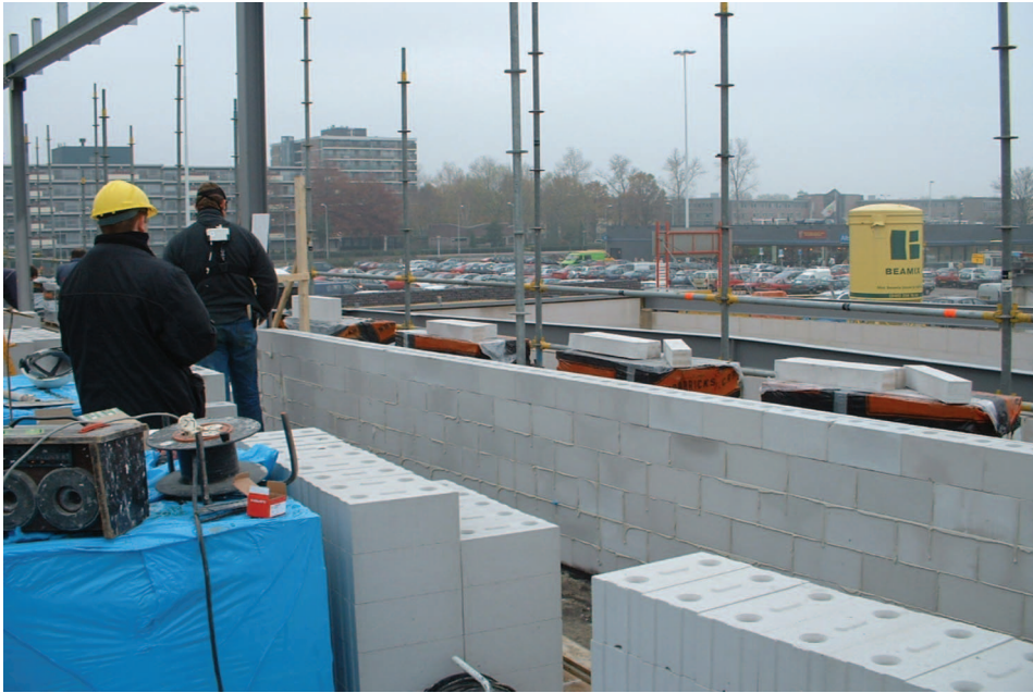
Figure 1. Field measurements of block mason building a wall consisting of 11 kg sandstone blocks.
